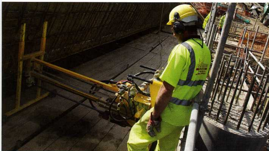
Right: The purpose-built 210B-42DD is drilling hundreds of horizontal holes of varying diameters and depths into the exposed sloping edges of the existing bridge deck and pier heads.
